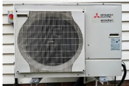
An air-source heat-pump fitted to the side of our house in Whaddon
